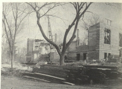
The front of the new library under construction, facing west on Linn Street
